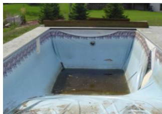
Damaged Vinyl Liner Low TA
